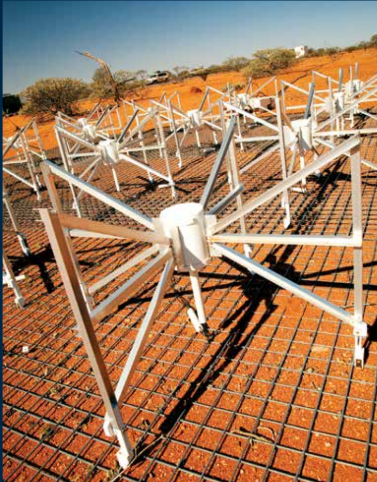
One Tile of 16 Murchison Widefield Array Antennas.
